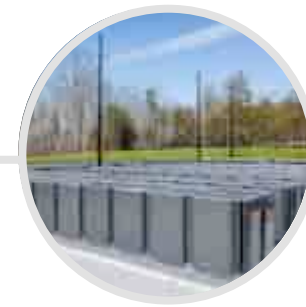
Power Center MWs – GWs
