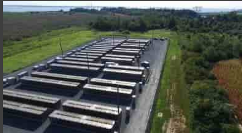
Delmarva Power, Delaware Utility Installation
