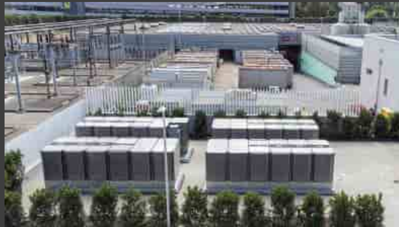
Ferrari, Maranello, Italy Packaged Energy Server
