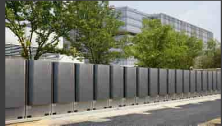
Intel, Bangalore, India Microgrid Installation
